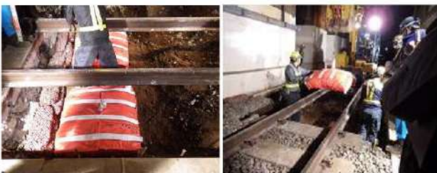
Photo-7: Mud pumping measures at Railway subgrade
