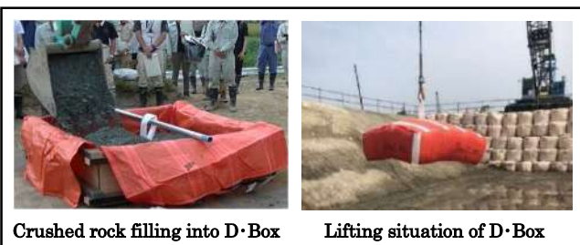
Photo -2: Filling of the intermediate material and a lifting status of D·Box
